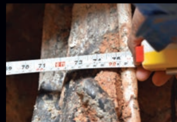
(Main, top to bottom) Great care is taken to ensure that the concrete wall for the investigation shaft does not affect the ground anchors; view of ground anchor from bottom; worker carefully exposing the ground anchor for investigation; each ground anchor's diameter is 150mm.
